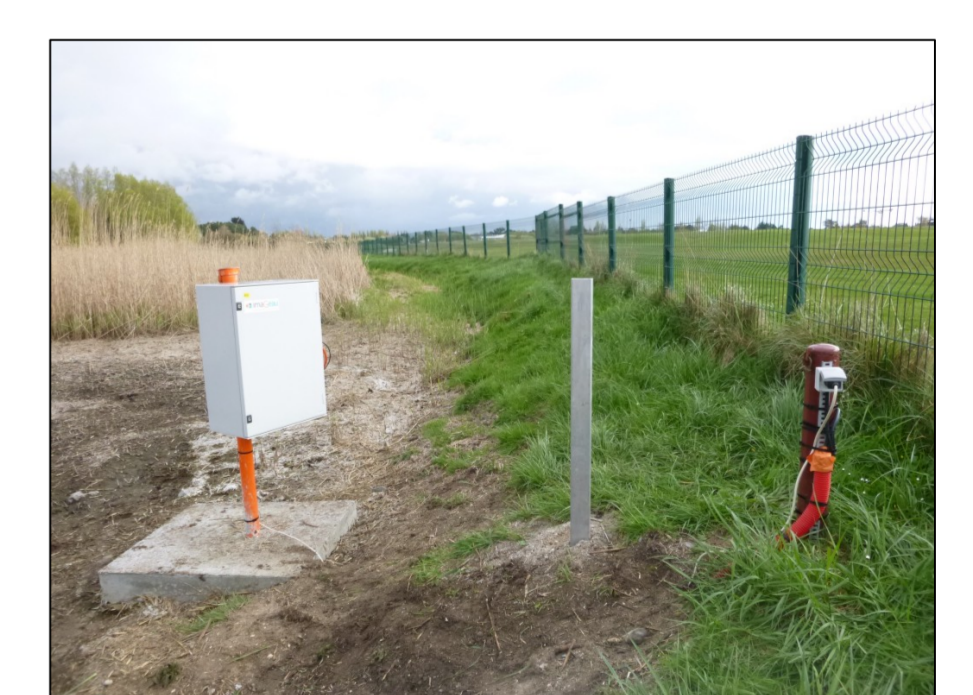
Acquisition Box outside
